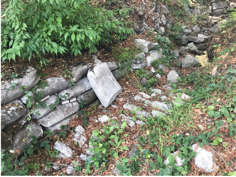
Figure 2. Failing sac-crete retaining wall along upper reach of Cerrito Creek within Blake Garden.
