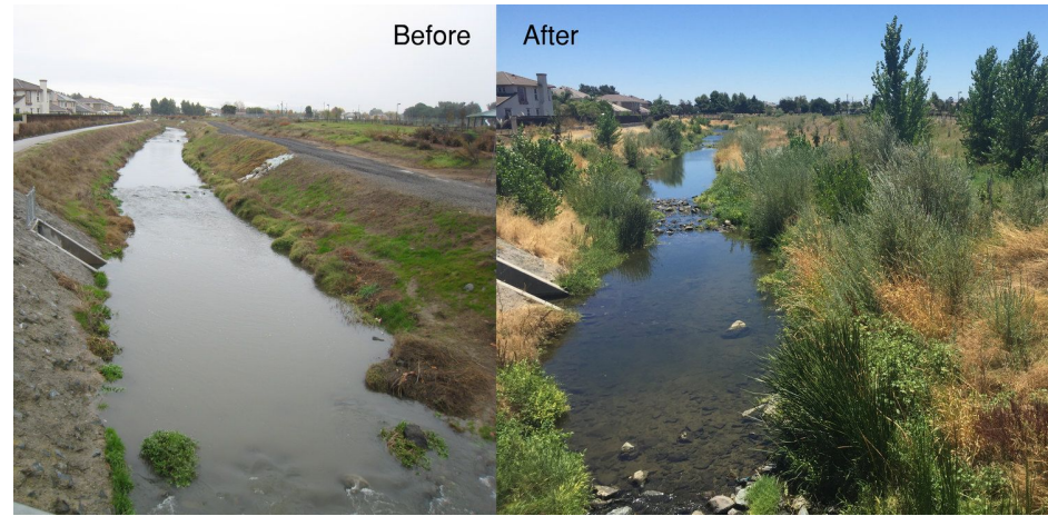
Example of urban stream restoration at Marsh Creek in Oakley, California, by Restoration Design Group
