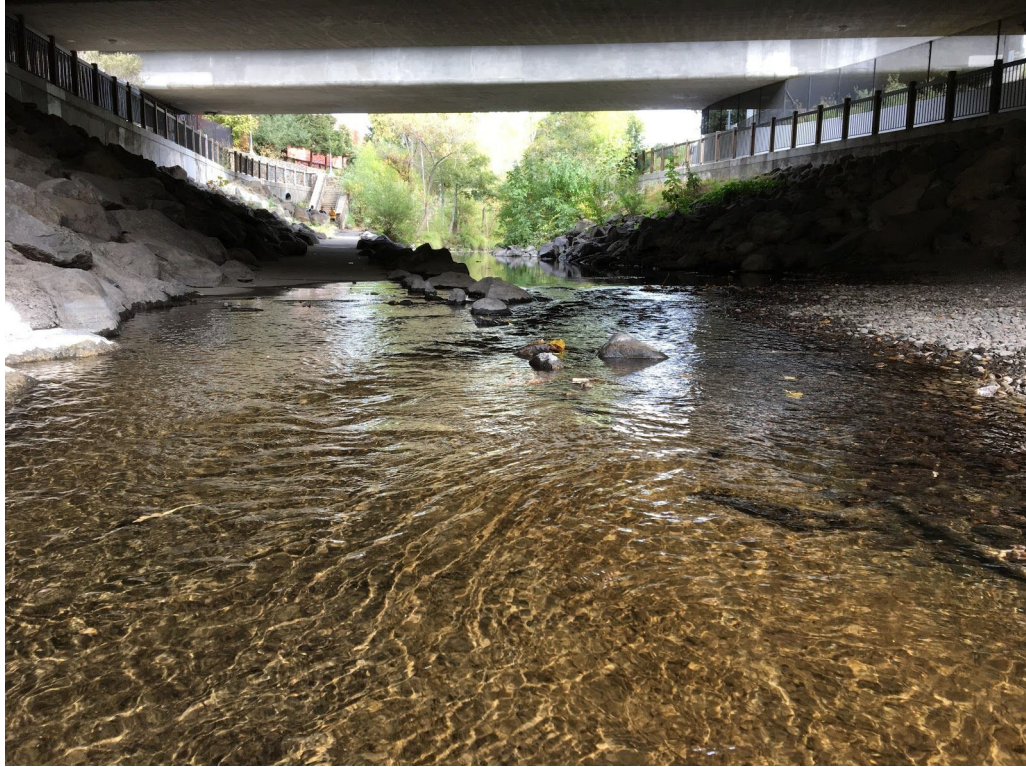
Photo 6: Location 4, shows shallow water flowing over sidewalk underneath Santa Ana Ave.
